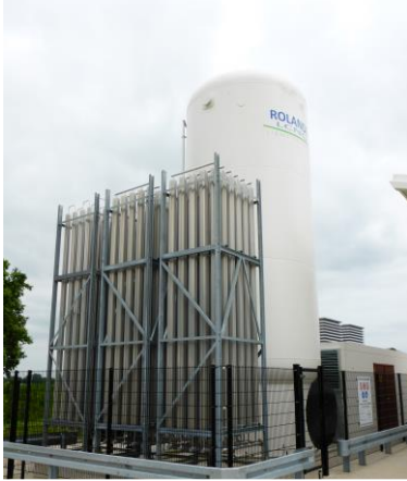
Storage tank with heat exchanger.
