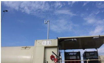
Supply installation blow-off pipe.
