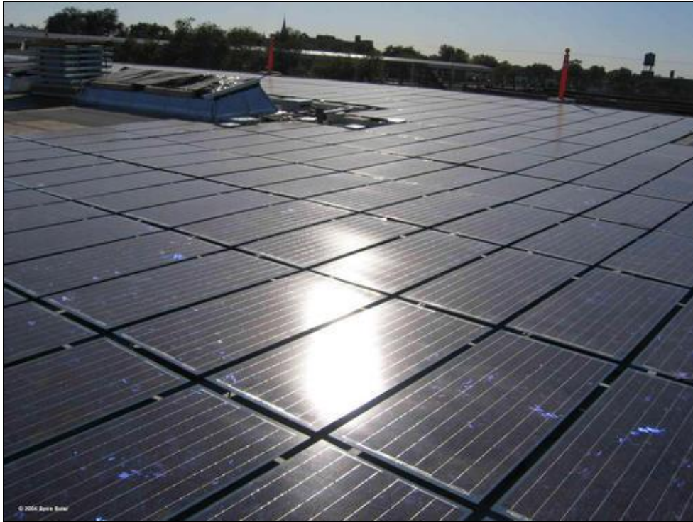
Figure 5-5: Example of a Large Photovoltaic Solar Power System on a Commercial Building (Photo courtesy of NREL Photographic Information Exchange)
