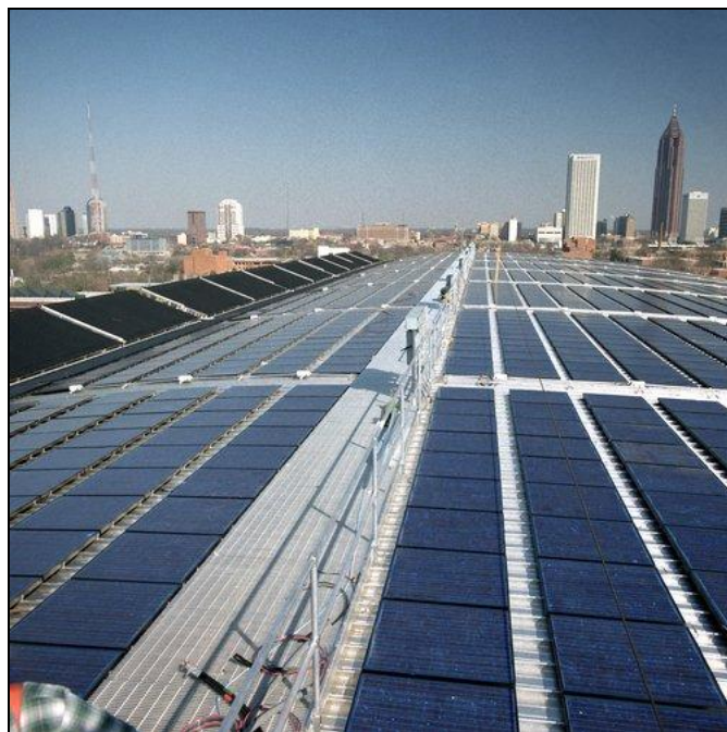
Figure 2-2: Rooftop Installation of Solar Thermal and PV Systems in Atlanta, GA (Photo courtesy of NREL Photographic Information Exchange)
