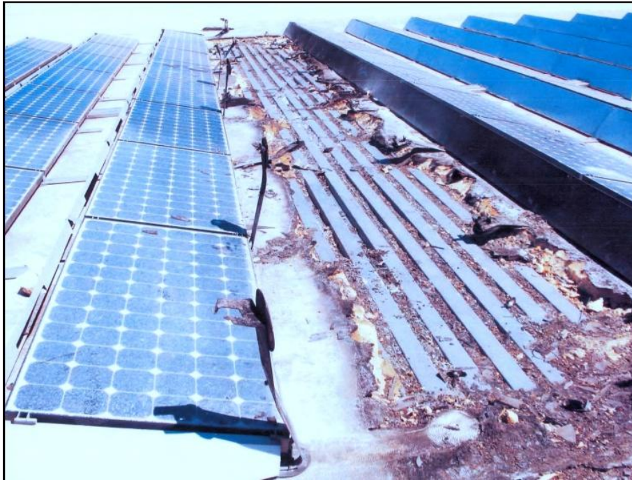
Figure 2-12: Fire-Damaged Array in April 2009 CA Incident 46
